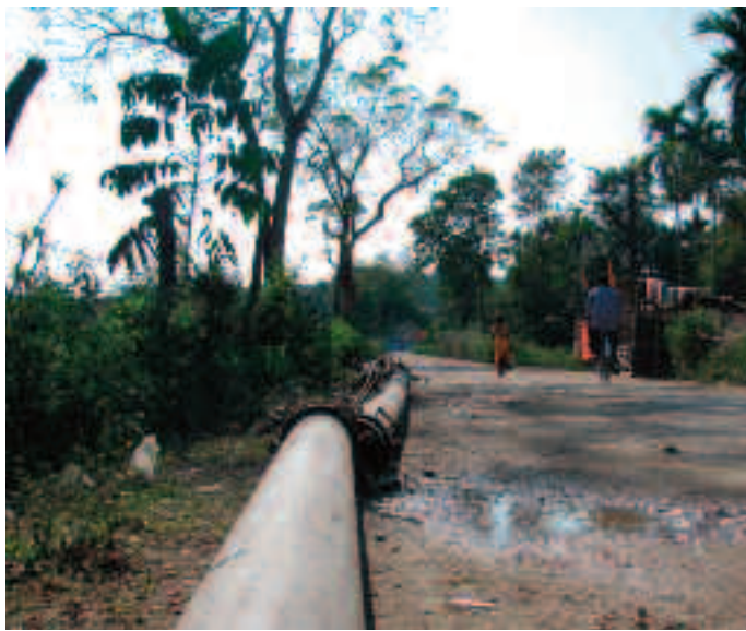
A broken pipeline, and hence disruption in water supply in the Terai and Dooars tea belt. Photo: Sayani Das
