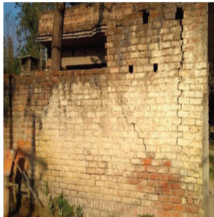
Cracks in the wall of Rizwan's house are getting bigger.
