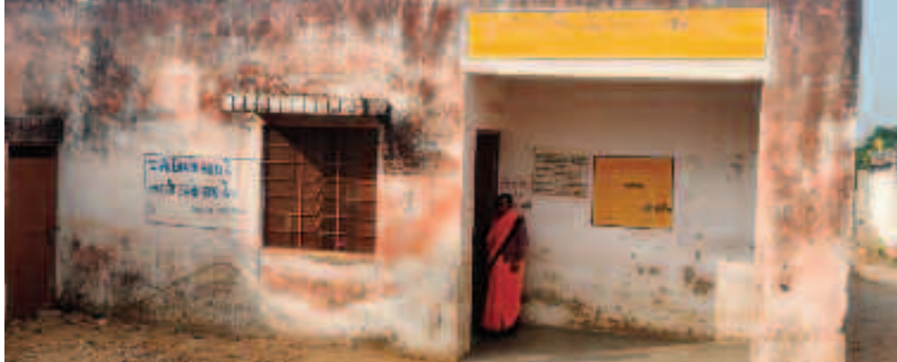
Sanjeeta Kawal at the decrepit anganwadi building in Motisar, Rajasthan.
