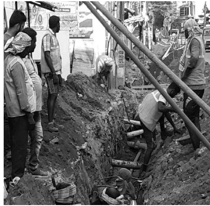
TNEB workers laying down underground electric cables at the Lake View Road, Adambakkam | RAHUL MANOJ
