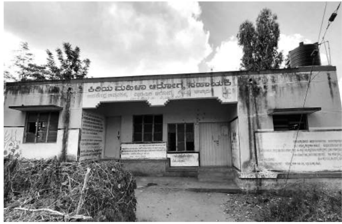
An abandoned PHC at Beemanahalli | SAMEER KULKARNI
