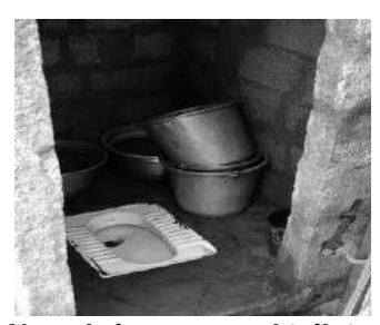
Vessels in an unused toilet | SUSMITHA ANN THOMAS
