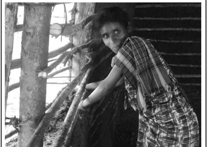
Bhagya single-handedly building a house to live in out of bamboo in Nagarhole forests | GOKUL GK
