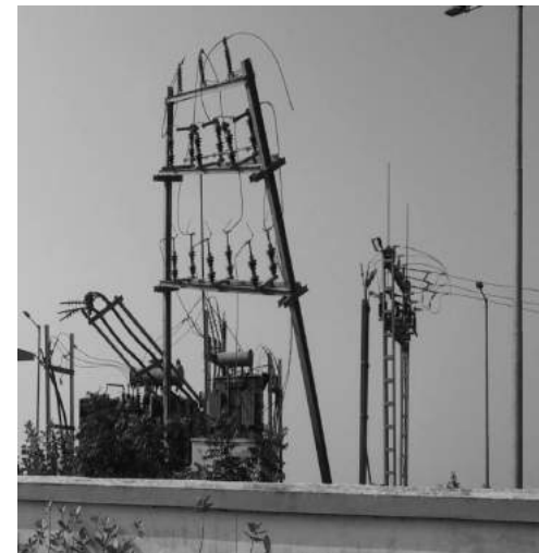
Damaged electricity poles right outside the Panasapada electricity office in the Brahmagiri block
