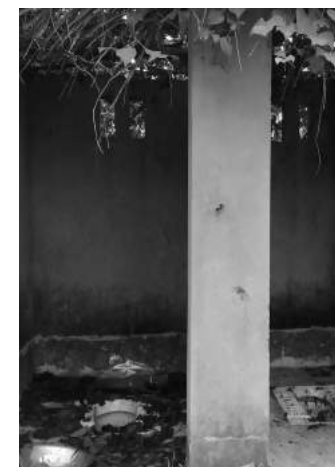
Fani-damaged toilets | MEGHA MALLICK
