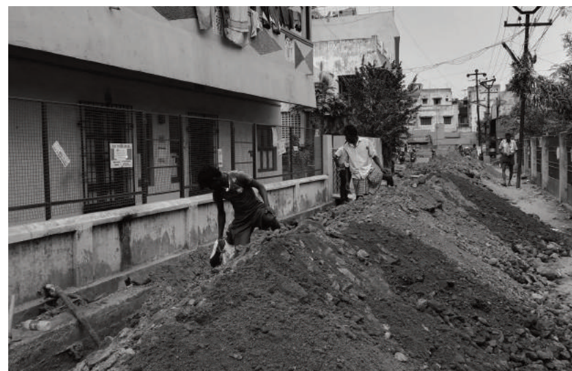
Water supply on Sarojini Street was disrupted after the road was dug up to lay cables for a mobile phone company. | ANSHITA BHATT
