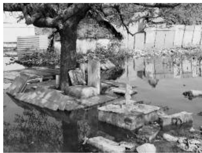
Hutment walls damaged by standing sewage | B PRADEEP
