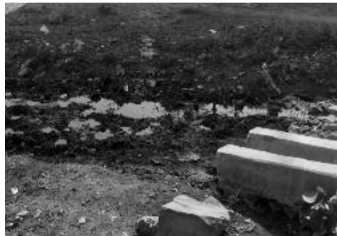
Improper drainage leading to stagnation | ADITHYA K
