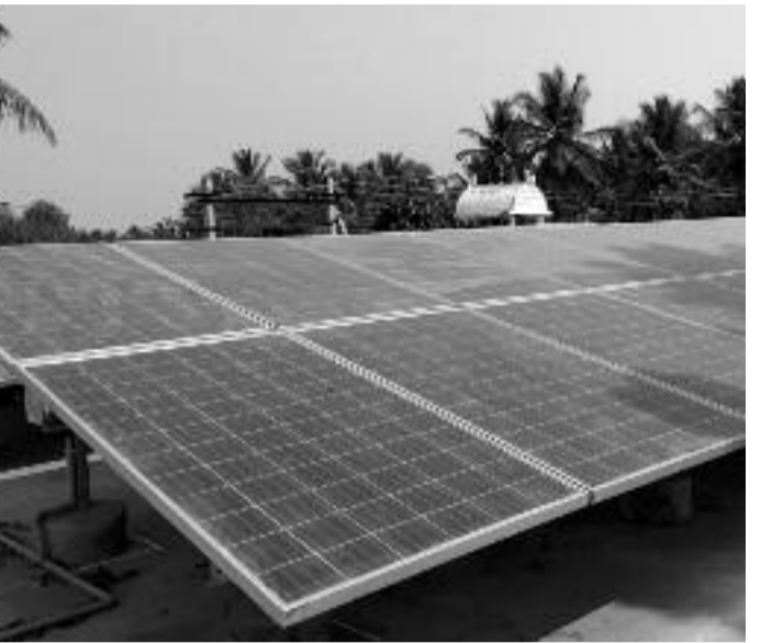
Solar panels installed at panchayat office in Sagare |AINDRILA PAUL
