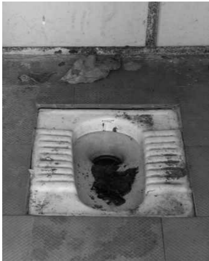
Well-constructed toilets remain unusable due to lack of proper water supply
